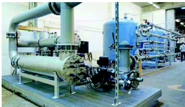
Foreground: Frame-mounted pumping unit with the UV disinfection system.
